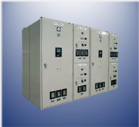
Medium-voltage metal enclosed switchgear
