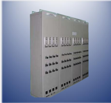
Transformers protection panel (154kV, 345kV, 765kV)
